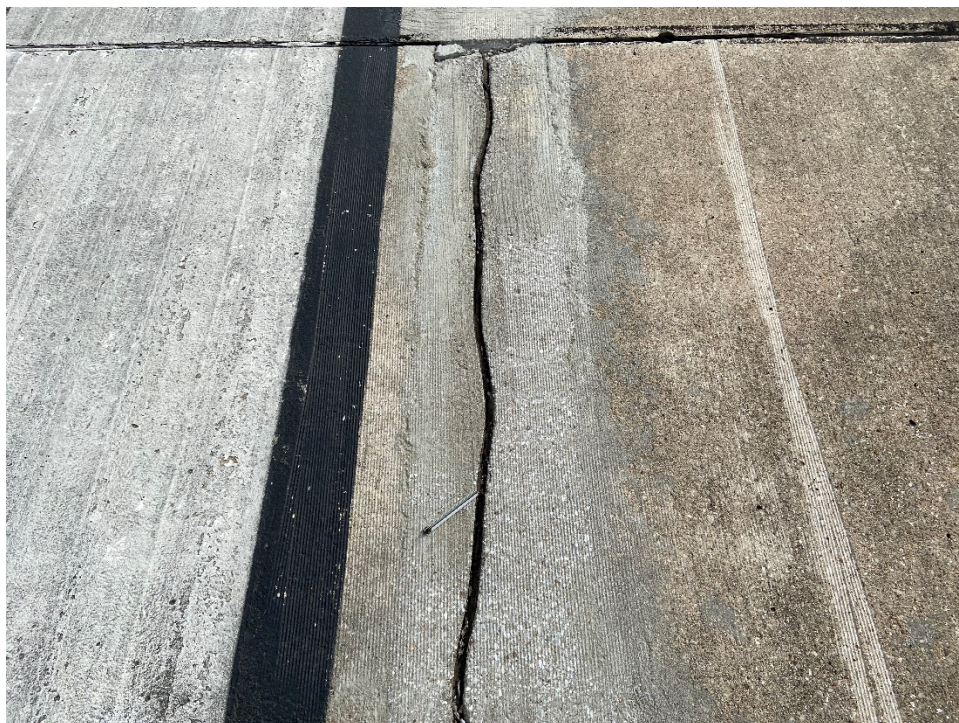
R11TI-01. Large Patching (Sample Unit No. 05).
