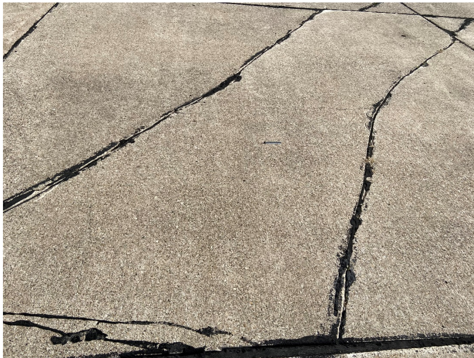
A01TI-01. Shattered Slab (Sample Unit No. 05).
