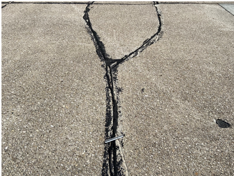
A01TI-01. LTD Cracking (Sample Unit No. 02).
