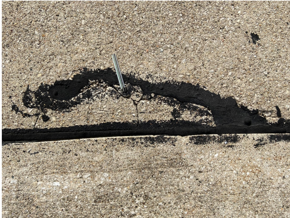
A01TI-01. Joint Spalling (Sample Unit No. 02).
