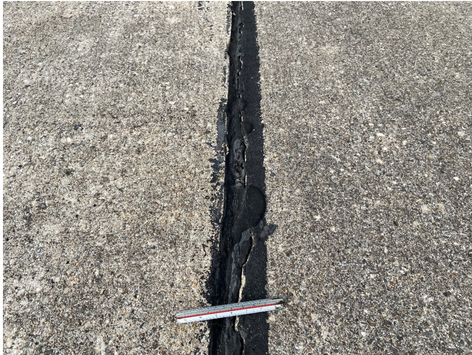
R11TI-01. LTD Cracking (Sample Unit No. 30).
