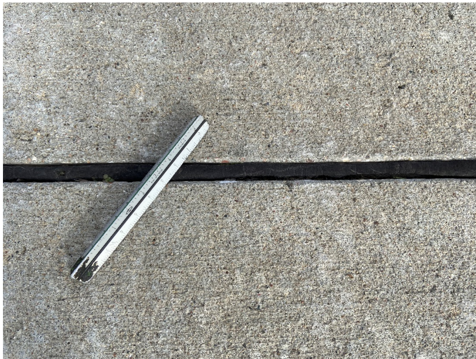
T01TI-02. Joint Seal Damage (Sample Unit No. 01).
