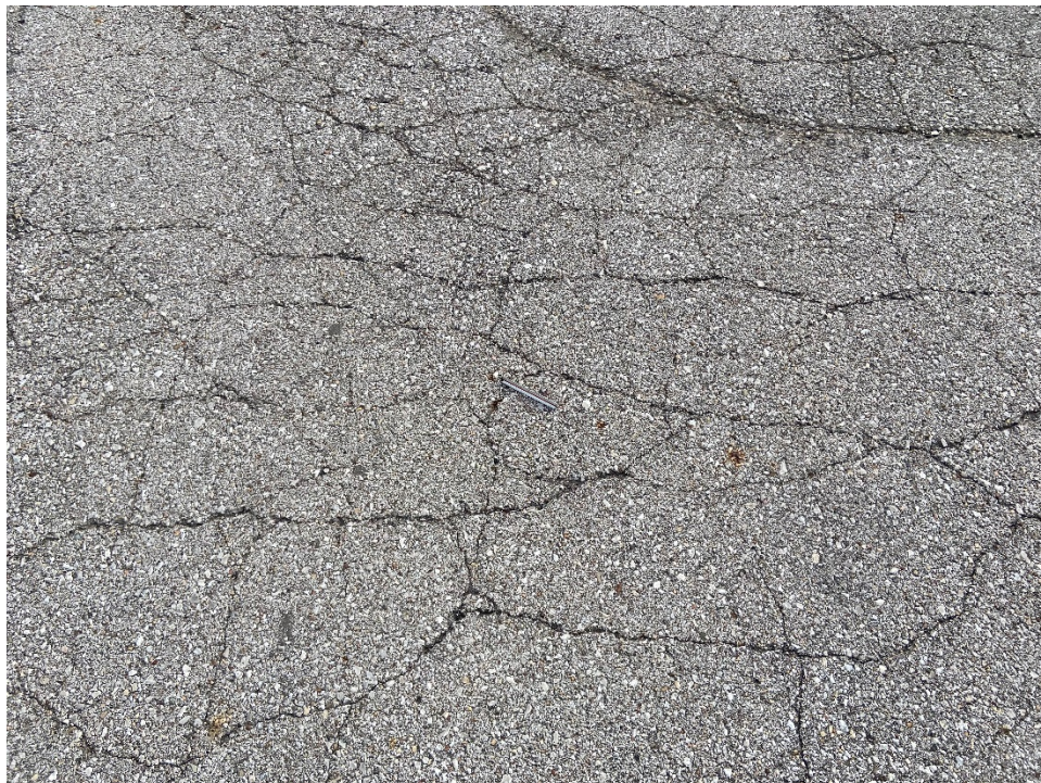
TH01TI-01. Alligator Cracking (Sample Unit No. 02).
