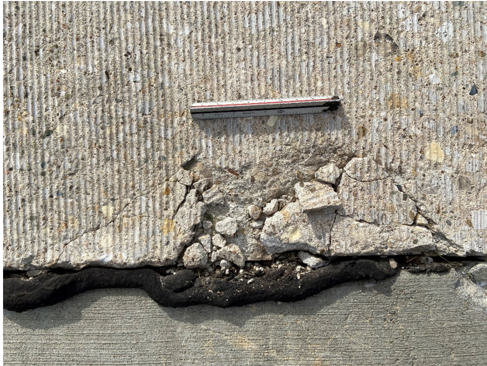
T01TI-03. Joint Spalling (Sample Unit No. 01) (2).
