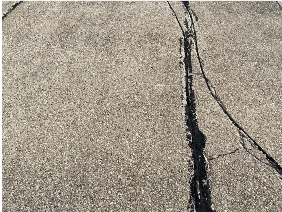
A01TI-01. Shattered Slab (Sample Unit No. 02).
