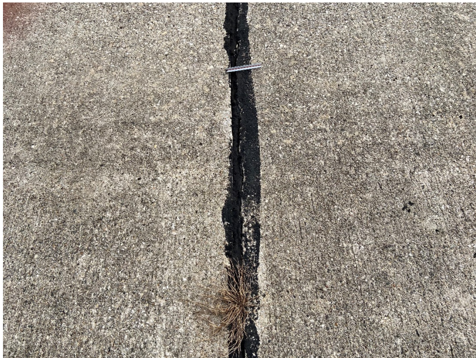
R11TI-01. LTD Cracking (Sample Unit No. 05).
