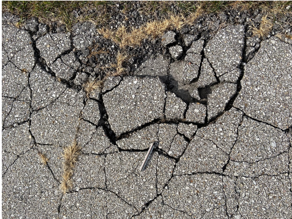
TH01TI-01. Alligator Cracking (Sample Unit No. 01).
