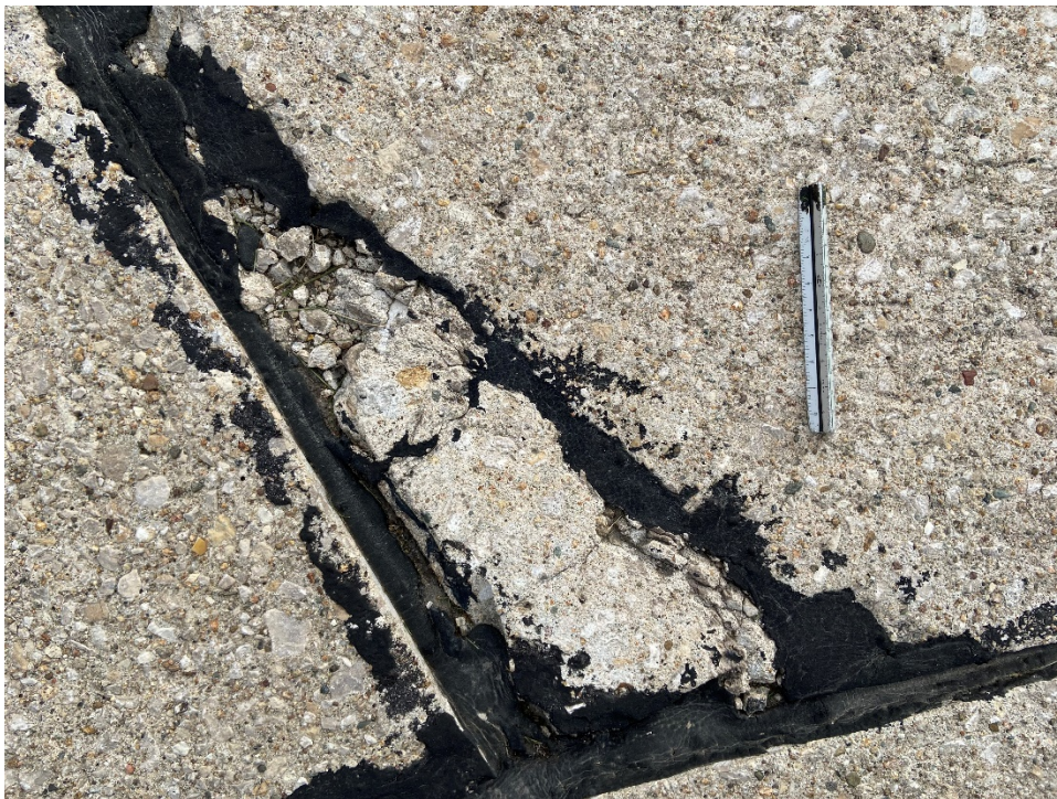
T01TI-03. Joint Spalling (Sample Unit No. 01) (1).
