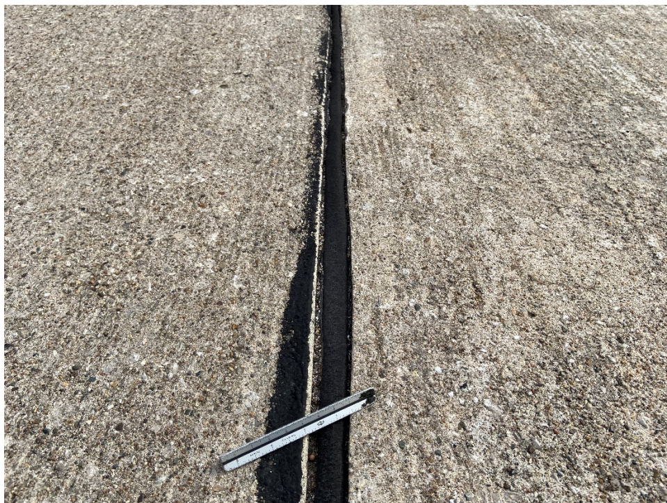
A01TI-01. Joint Seal Damage (Sample Unit No. 03).
