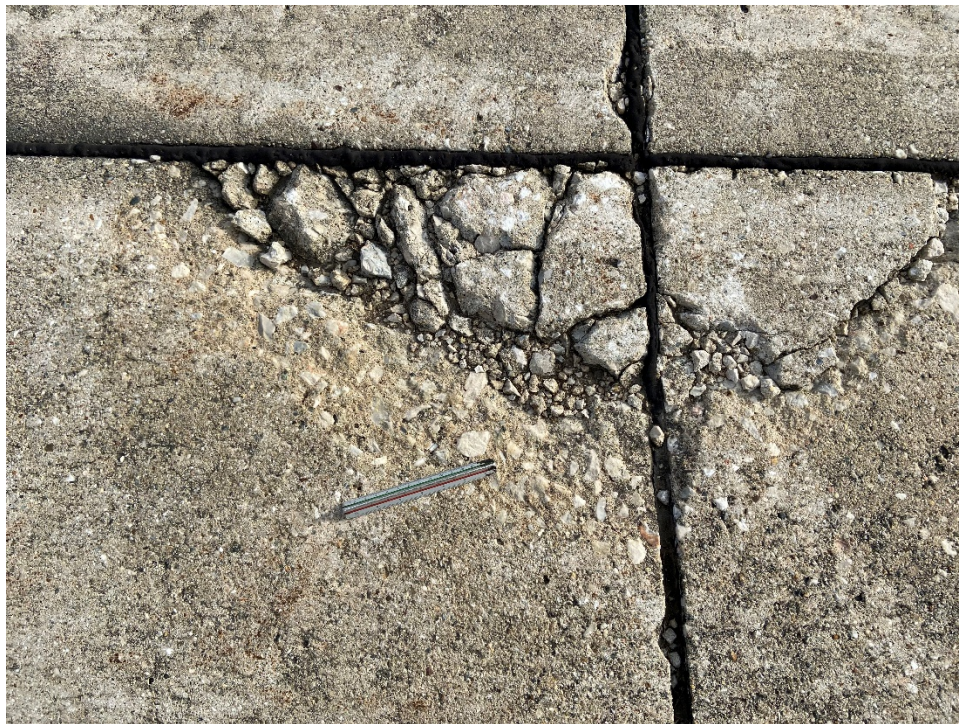
A01WU-04. Corner Spalling (Sample Unit No. 05).
