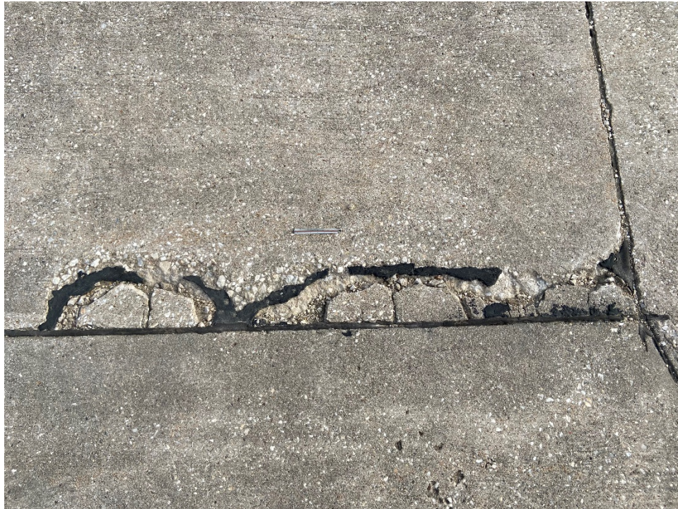
A01WU-01. Joint Spalling (Sample Unit No. 02) (2).
