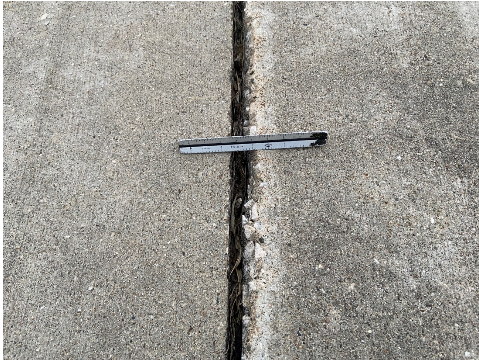
R17WU-04. Joint Seal Damage (Sample Unit No. 01).
