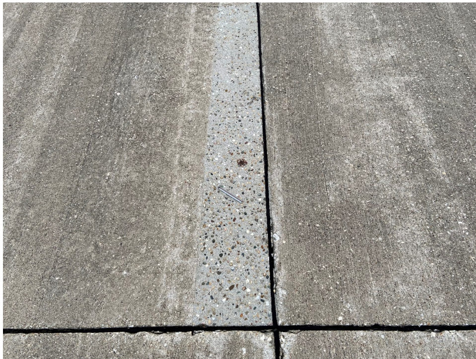
R17WU-01. Large Patching (Sample Unit No. 04).
