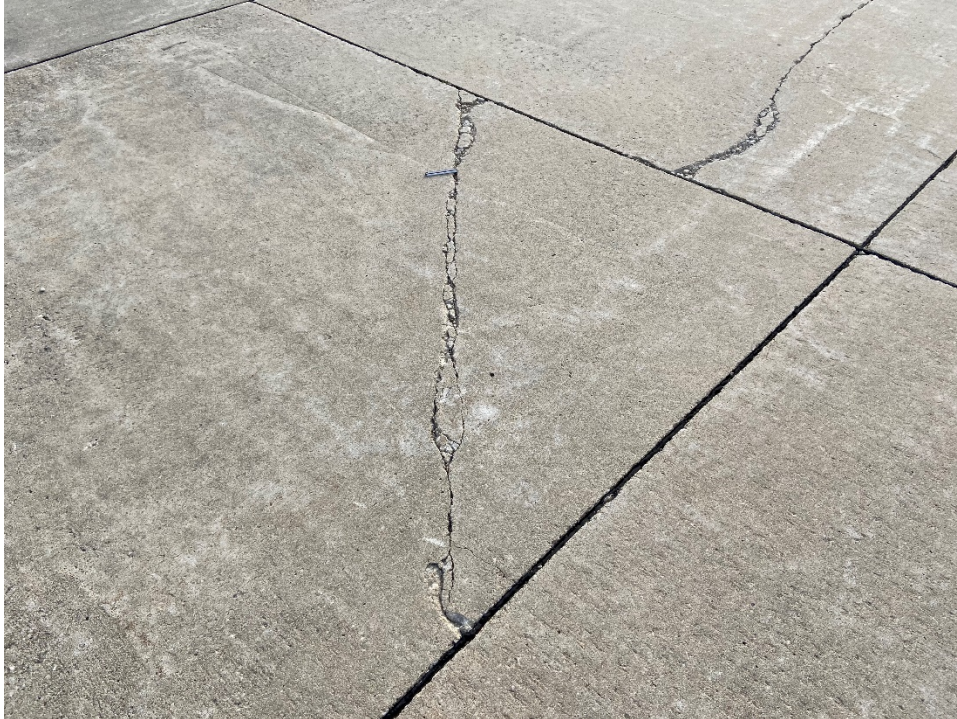
A01WU-04. LTD Cracking (Sample Unit No. 01).
