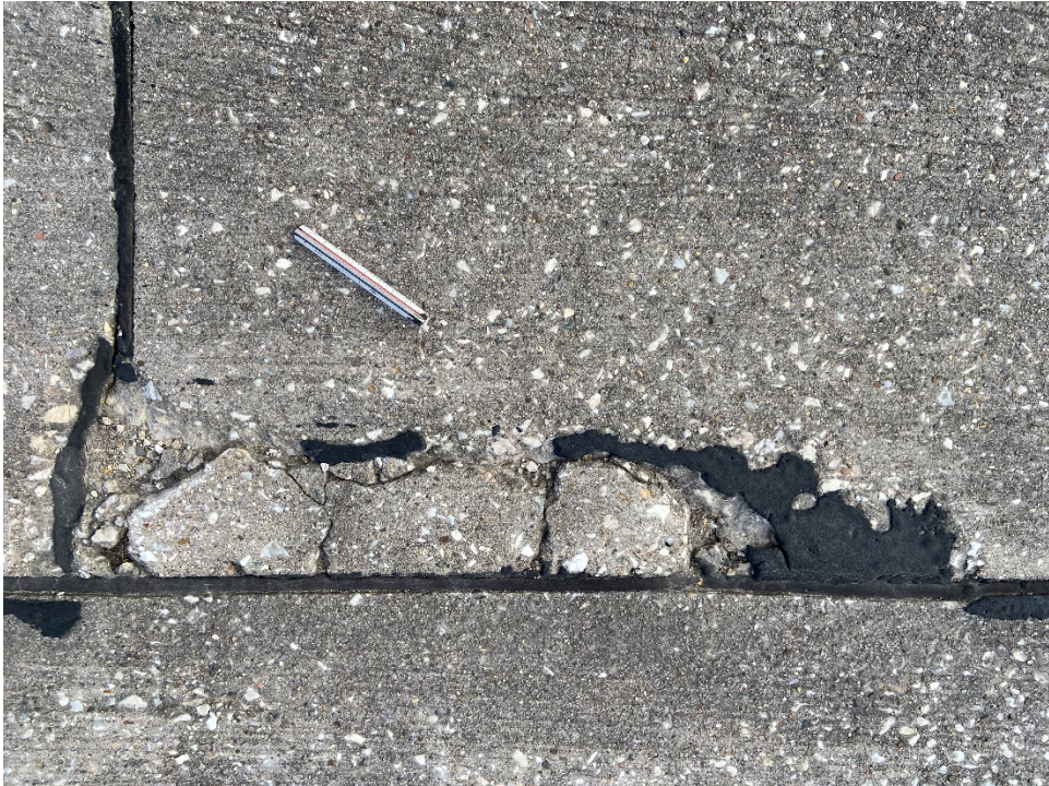
A01WU-01. Joint Spalling (Sample Unit No. 02) (1).
