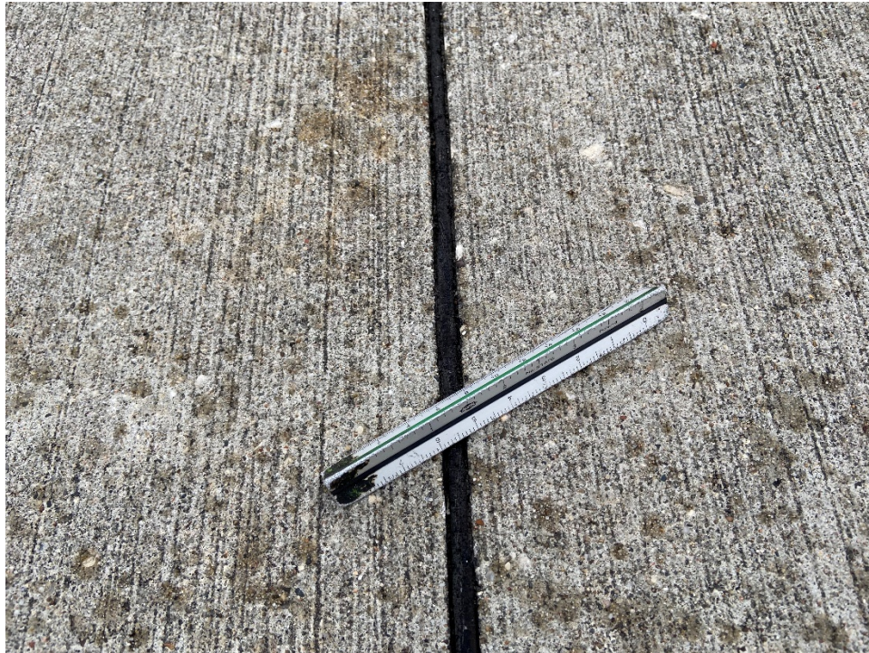
R17WU-03. Joint Seal Damage (Sample Unit No. 39).
