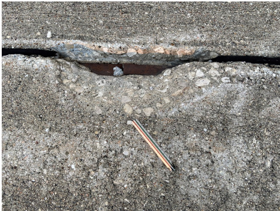
R17WU-01. Joint Spalling (Sample Unit No. 04).
