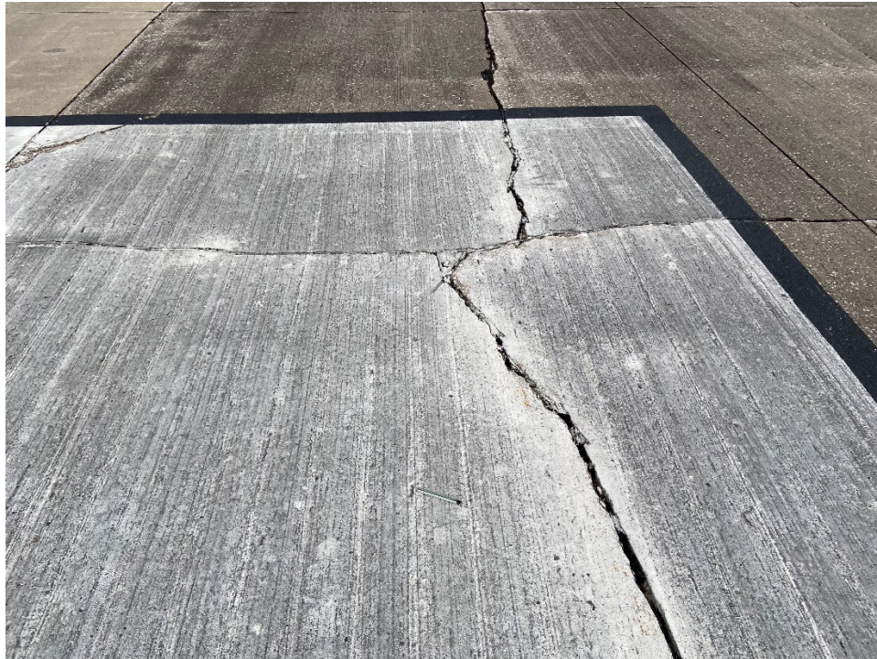
R17WU-02. Shattered Slab (Sample Unit No. 03).
