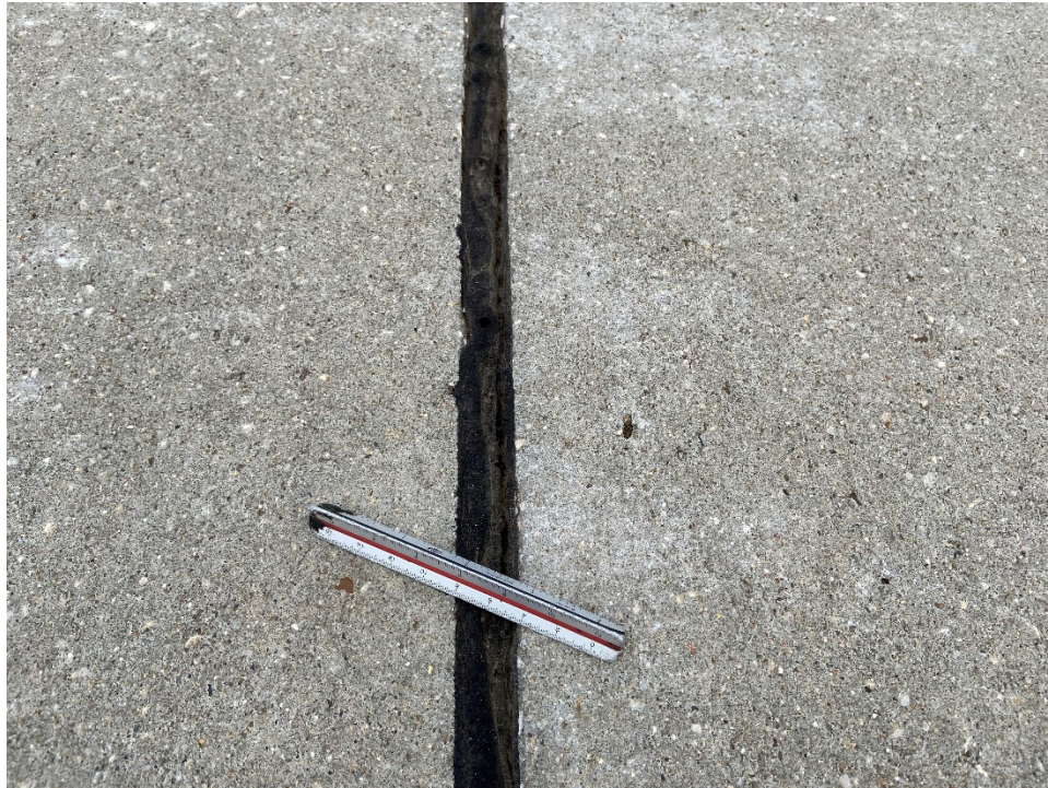
T01WU-01. Joint Seal Damage (Sample Unit No. 01).
