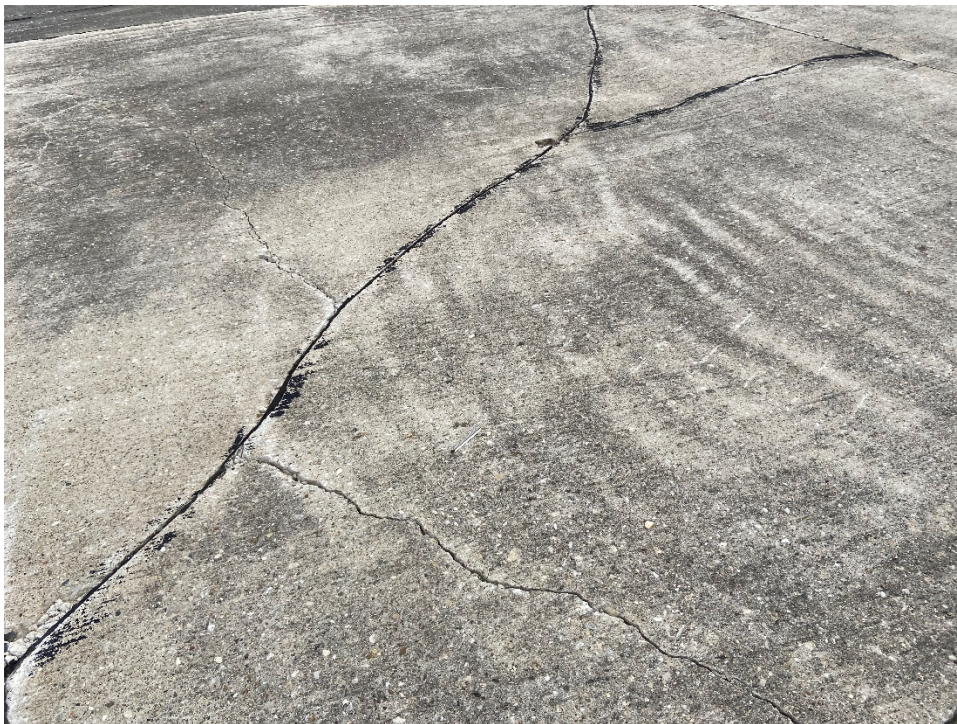
A01WU-02. Shattered Slab (Sample Unit No. 01).
