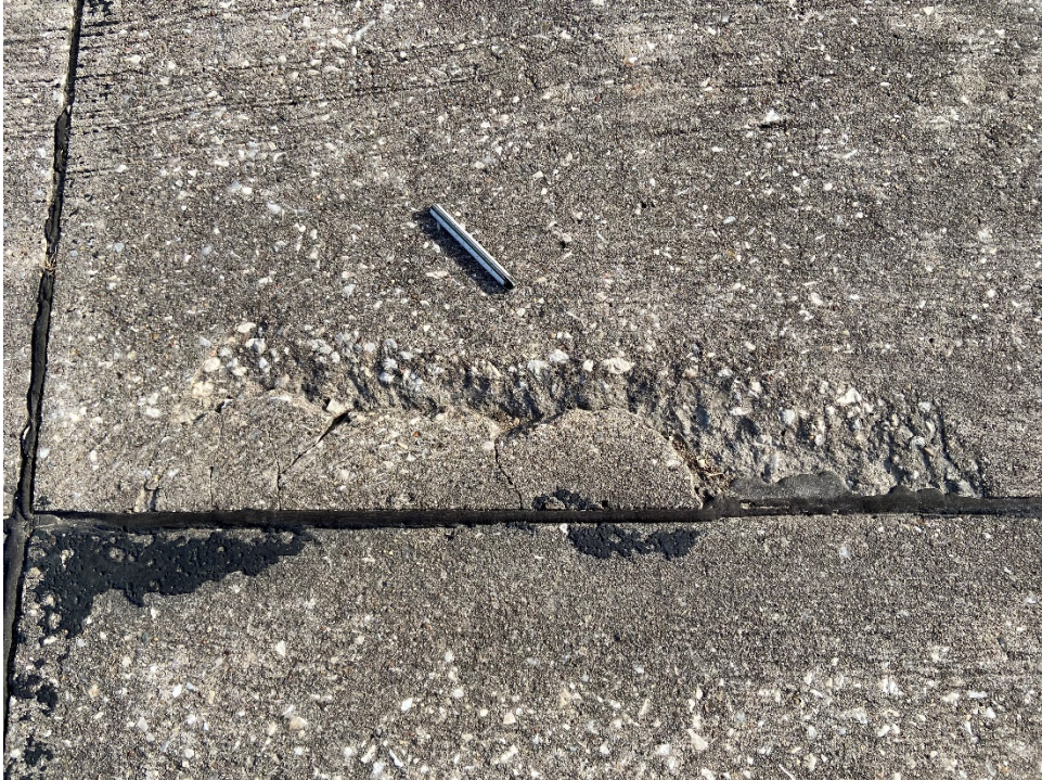
A01WU-01. Joint Spalling (Sample Unit No. 01).
