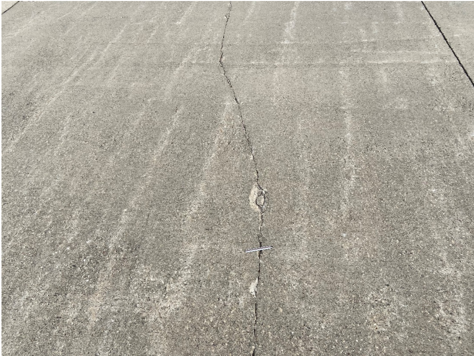
TH01WU-01. LTD Cracking (Sample Unit No. 01).
