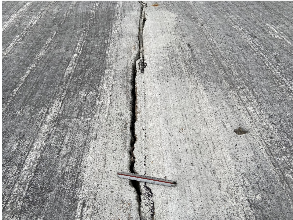
R17WU-02. LTD Cracking (Sample Unit No. 03).
