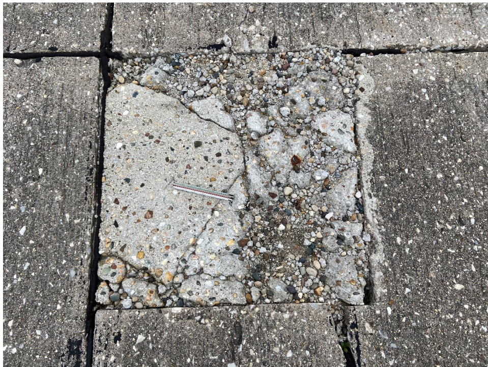
R17WU-02. Small Patching (Sample Unit No. 12).
