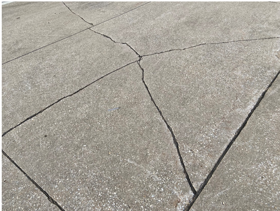
A01WU-01. Shattered Slab (Sample Unit No. 02).
