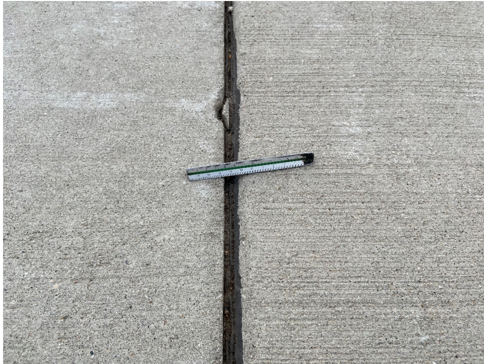
A01WU-05. Joint Seal Damage (Sample Unit No. 01).
