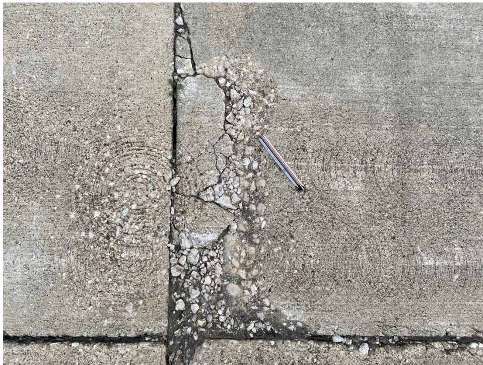
R17WU-04. Joint Spalling (Sample Unit No. 02).
