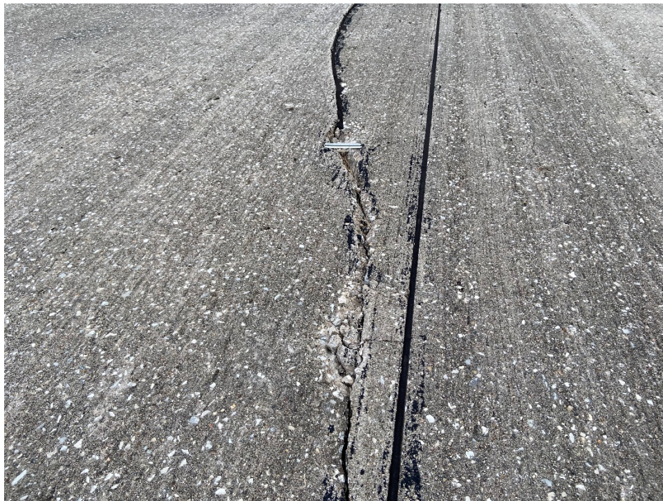
R17WU-02. LTD Cracking (Sample Unit No. 16).
