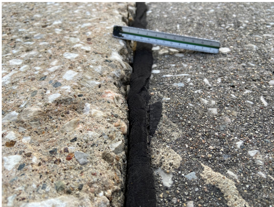
A01WU-01. Faulting (Sample Unit No. 02).
