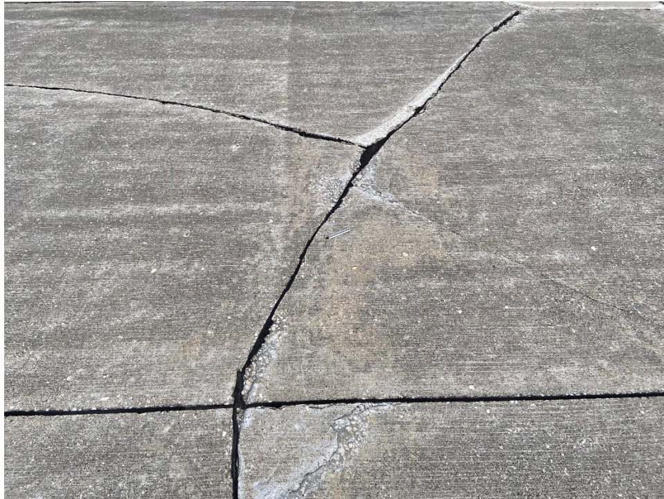
R17WU-01. Shattered Slab (Sample Unit No. 13).
