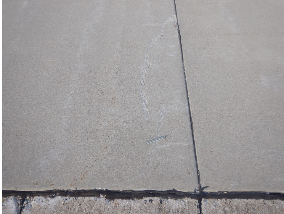
A01WU-05. Joint Spalling (Sample Unit No. 03).
