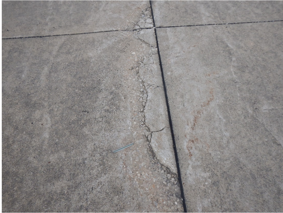
A01WU-04. Joint Spalling (Sample Unit No. 05).
