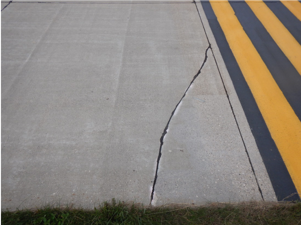
R17WU-04. LTD Cracking (Sample Unit No. 01).
