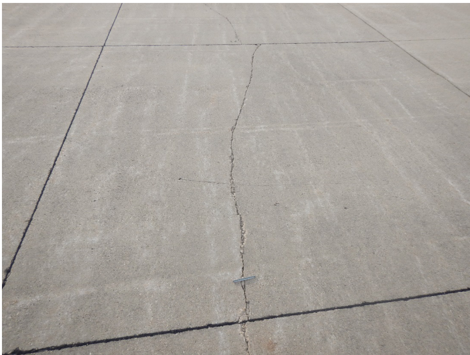
TH01WU-01. LTD Cracking (Sample Unit No. 01).
