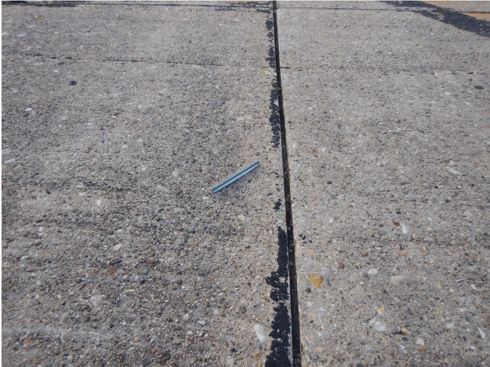
A01WU-02. Joint Seal Damage (Sample Unit No. 01).
