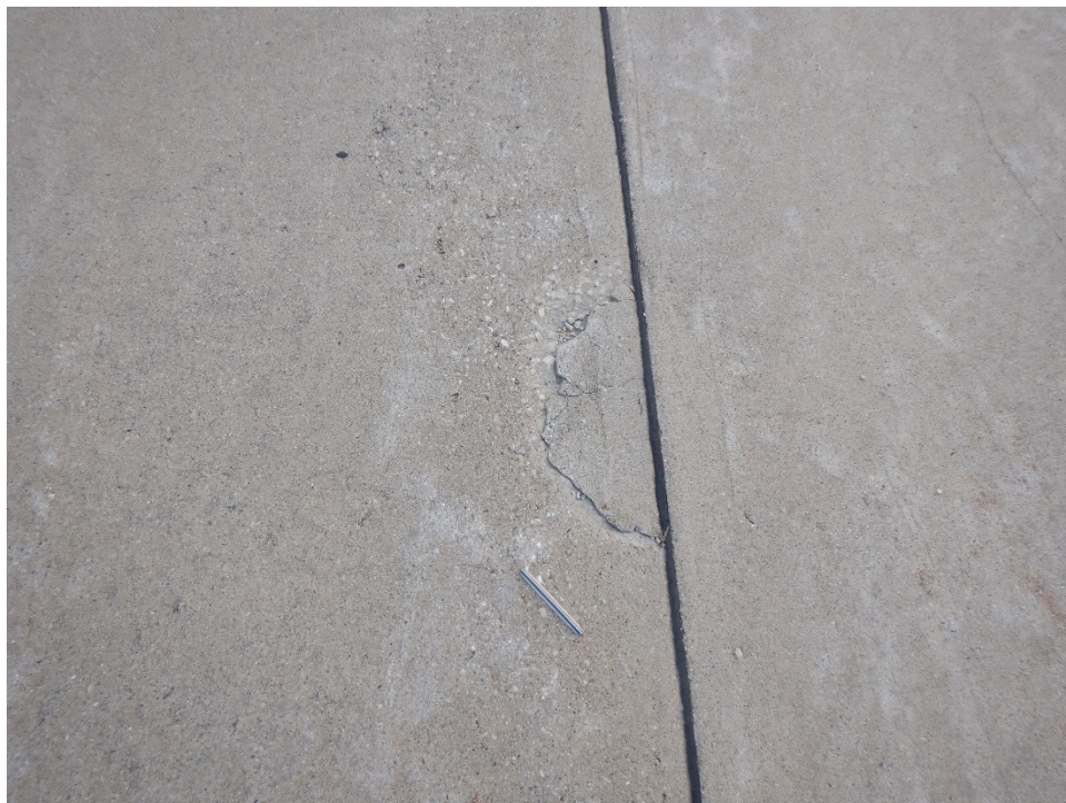
A01WU-03. Joint Spalling (Sample Unit No. 02).
