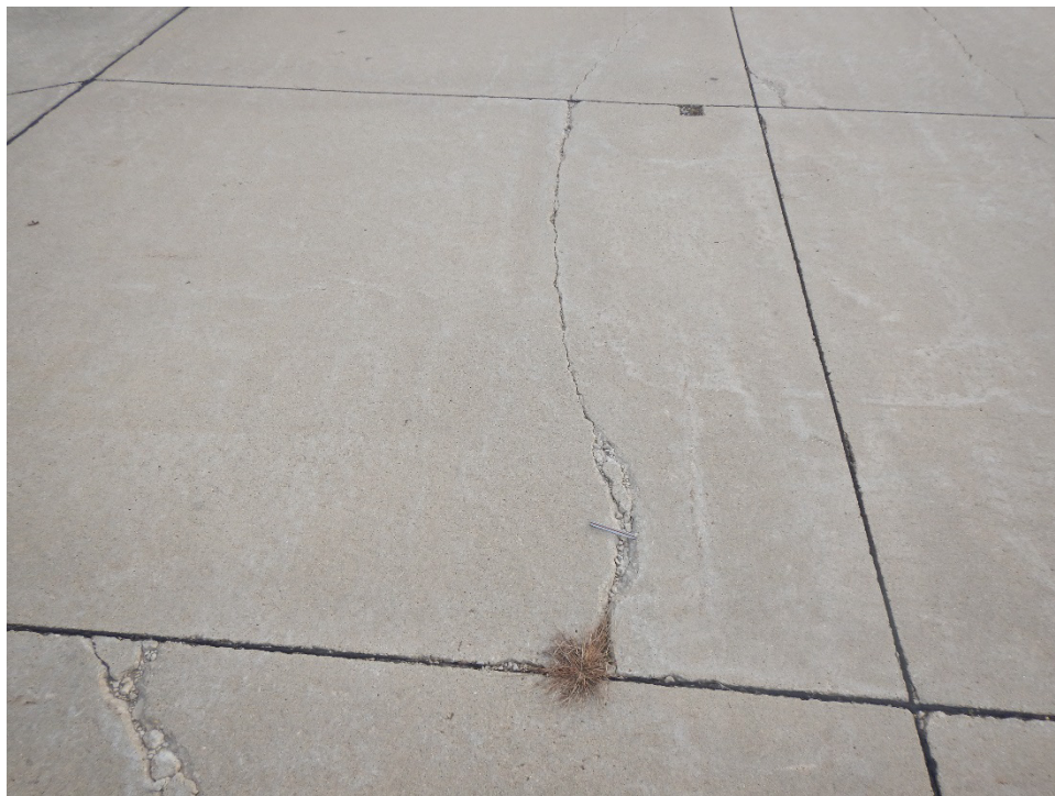
A01WU-04. LTD Cracking (Sample Unit No. 01).
