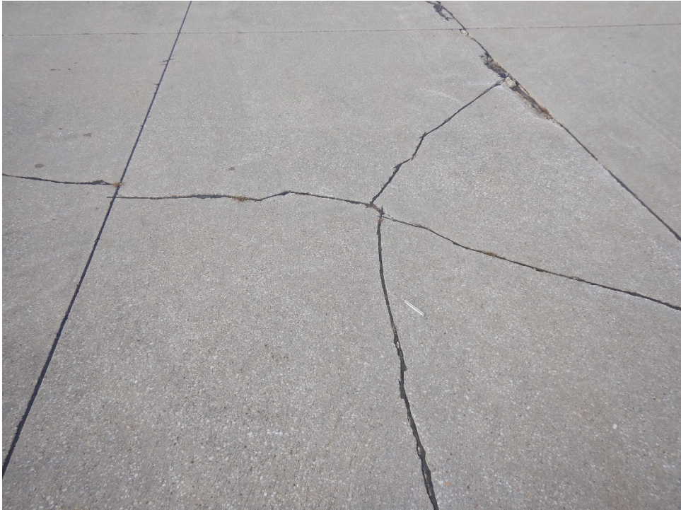
A01WU-01. Shattered Slab (Sample Unit No. 02).
