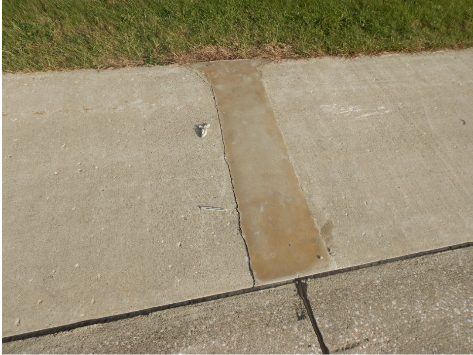
R17WU-03. Large Patching (Sample Unit No. 22).
