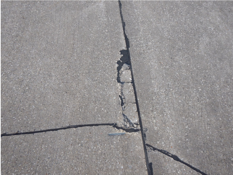
A01WU-01. Joint Spalling (Sample Unit No. 01).
