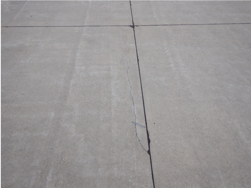
R17WU-04. Joint Spalling (Sample Unit No. 01).
