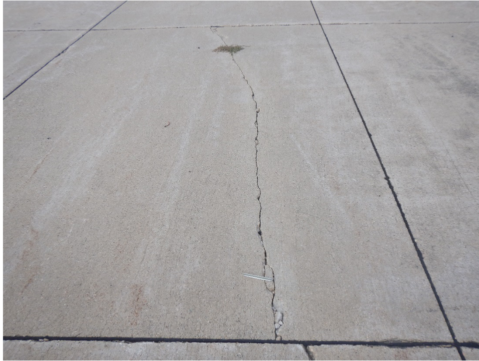
A01WU-03. LTD Cracking (Sample Unit No. 01).
