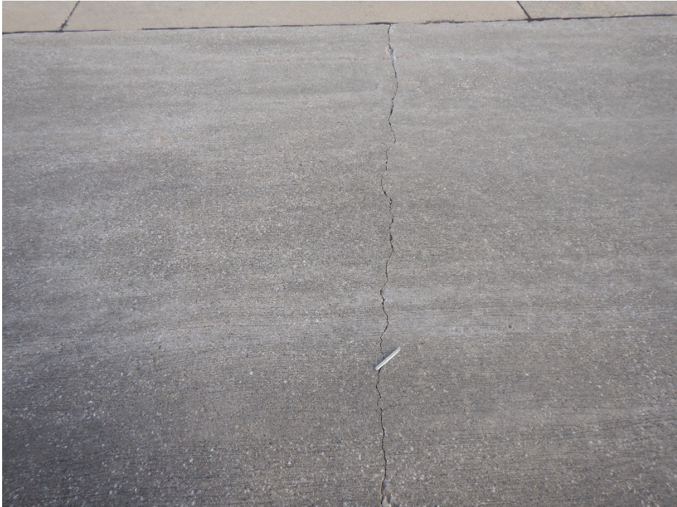
A01WU-01. LTD Cracking (Sample Unit No. 01).
