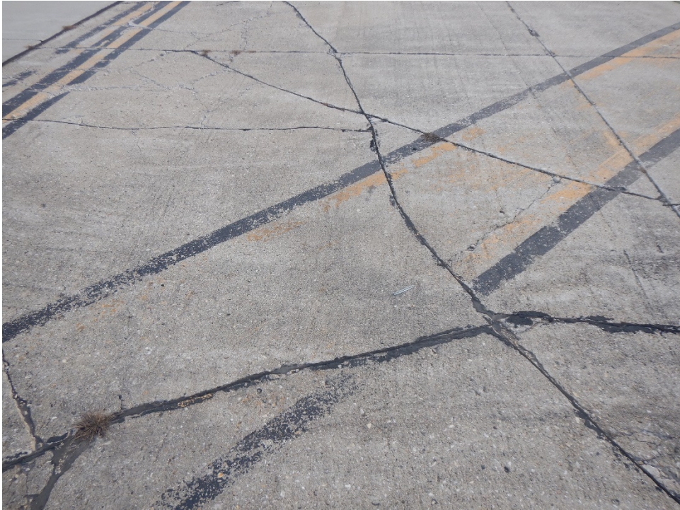
A01WU-02. Shattered Slab (Sample Unit No. 01).
