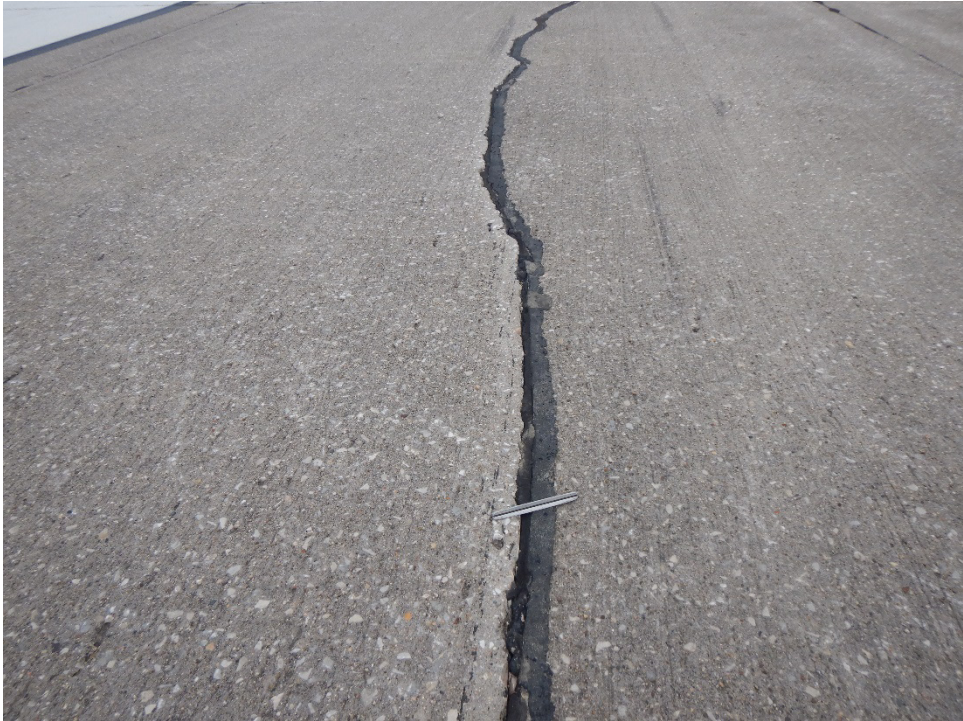
R17WU-02. LTD Cracking (Sample Unit No. 03).
