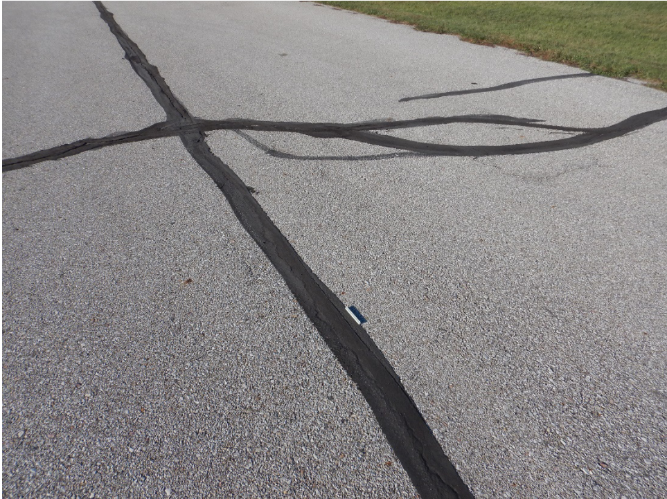
A01WI-01. L&T Cracking (Sample Unit No. 05).
