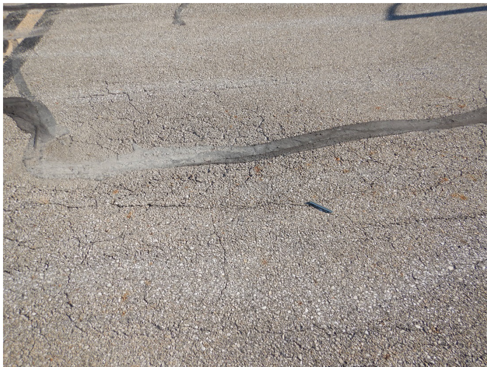
TH01WI-01. Alligator Cracking (Sample Unit No. 05).
