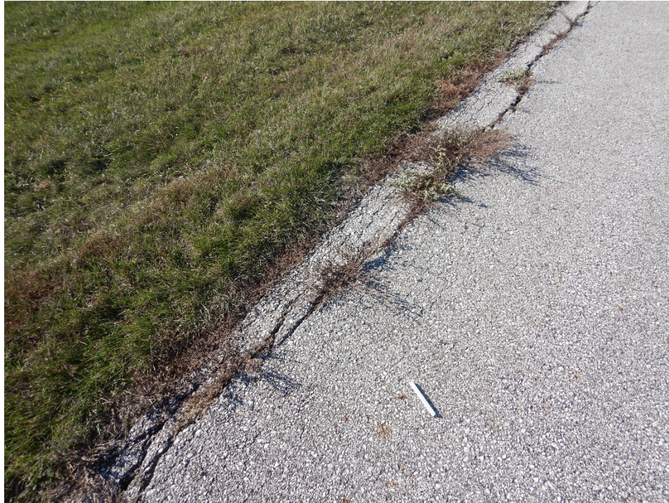
R14WI-01. Alligator Cracking (Sample Unit No. 16).
