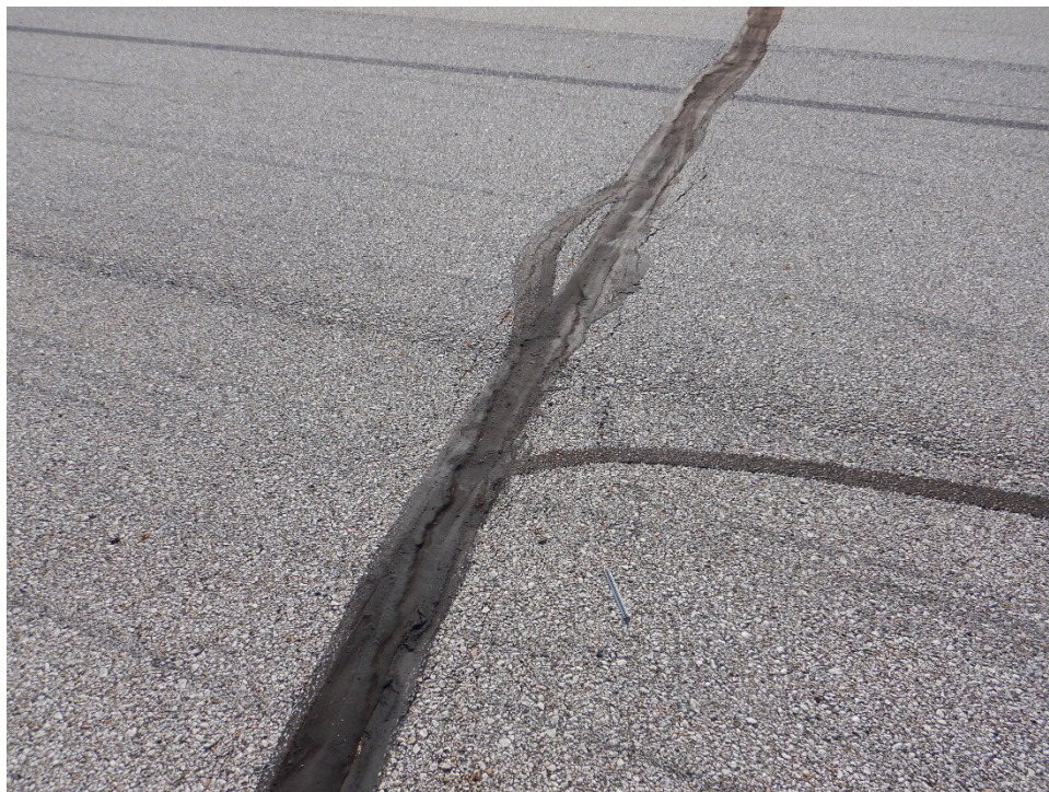
R14WI-01. L&T Cracking (Sample Unit No. 24).
