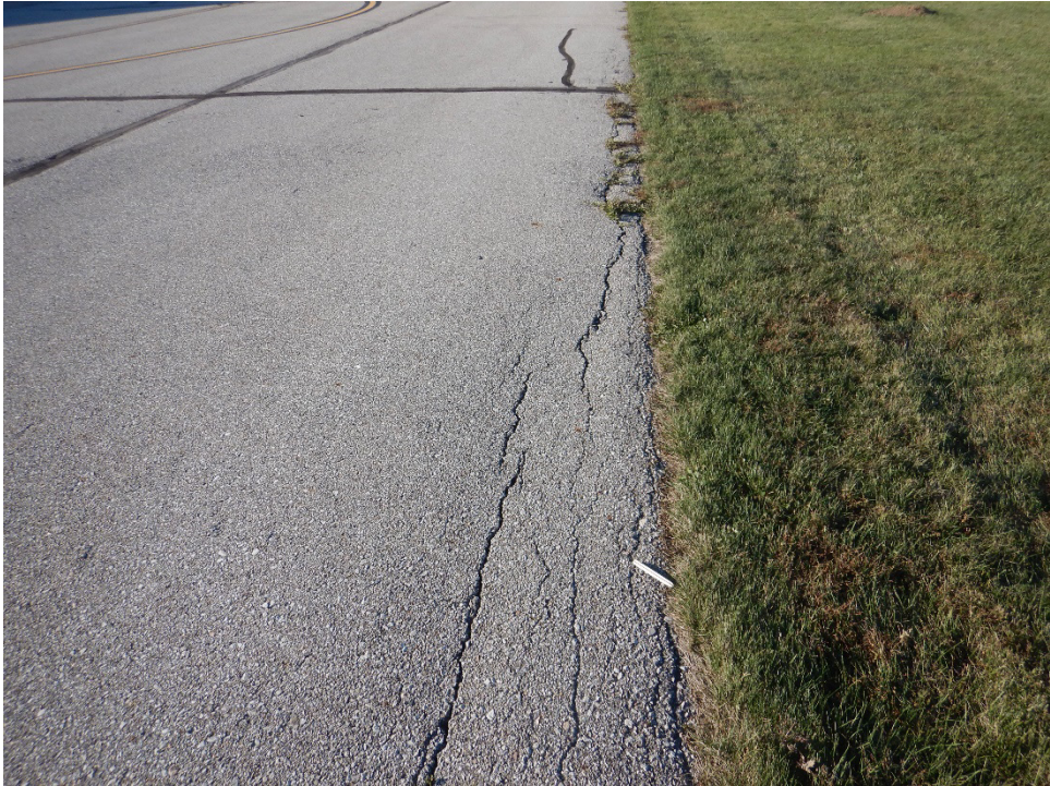
A01WI-01. Alligator Cracking (Sample Unit No. 06).
