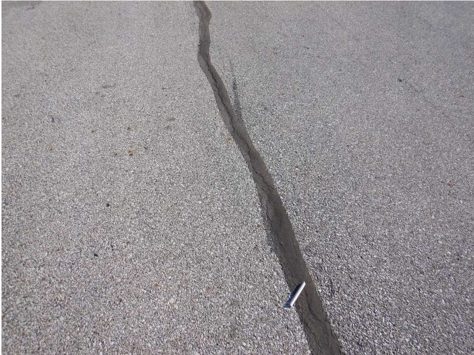
TH01WI-02. L&T Cracking (Sample Unit No. 02).
