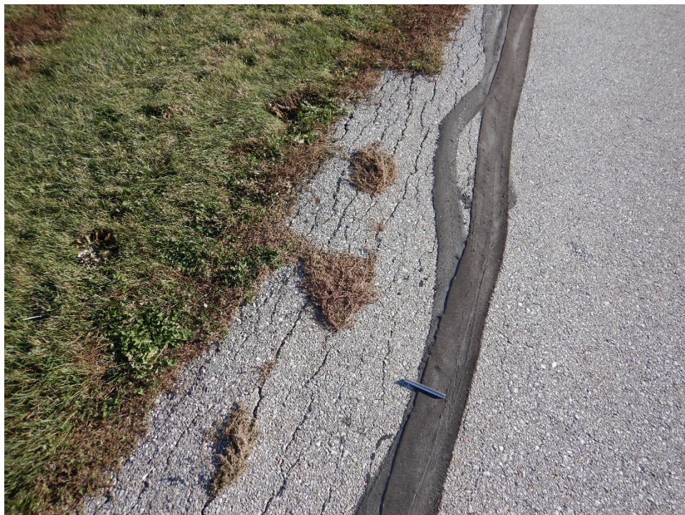
T01WI-01. Alligator Cracking (Sample Unit No. 01).
