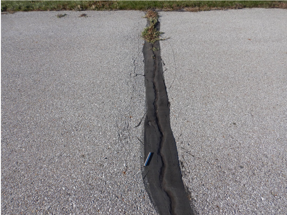
T02WI-01. L&T Cracking (Sample Unit No. 01).
