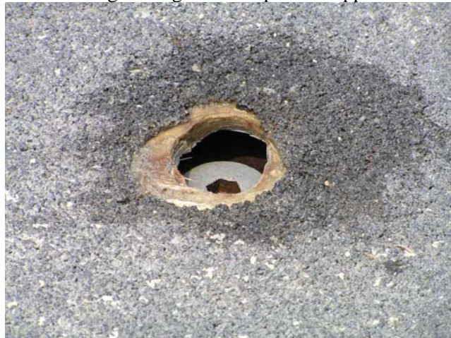
Figure 35. Delamination of top layer of FRP at a lifting lug location.
