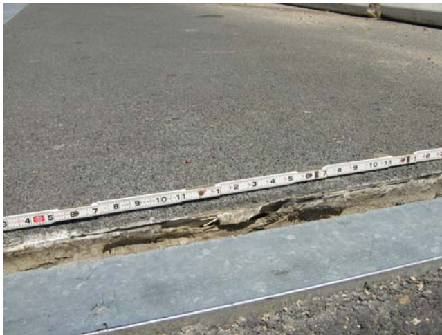
Figure 34. Damage at edge of deck panel at approach abutment.
