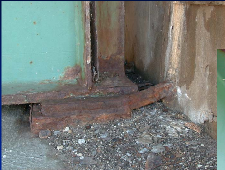
Corroded abutment bearing
