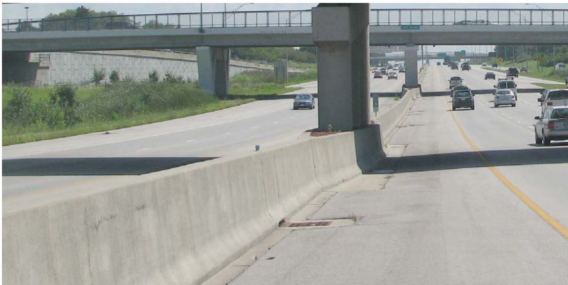
Figure 4: Permanent concrete barrier example.
