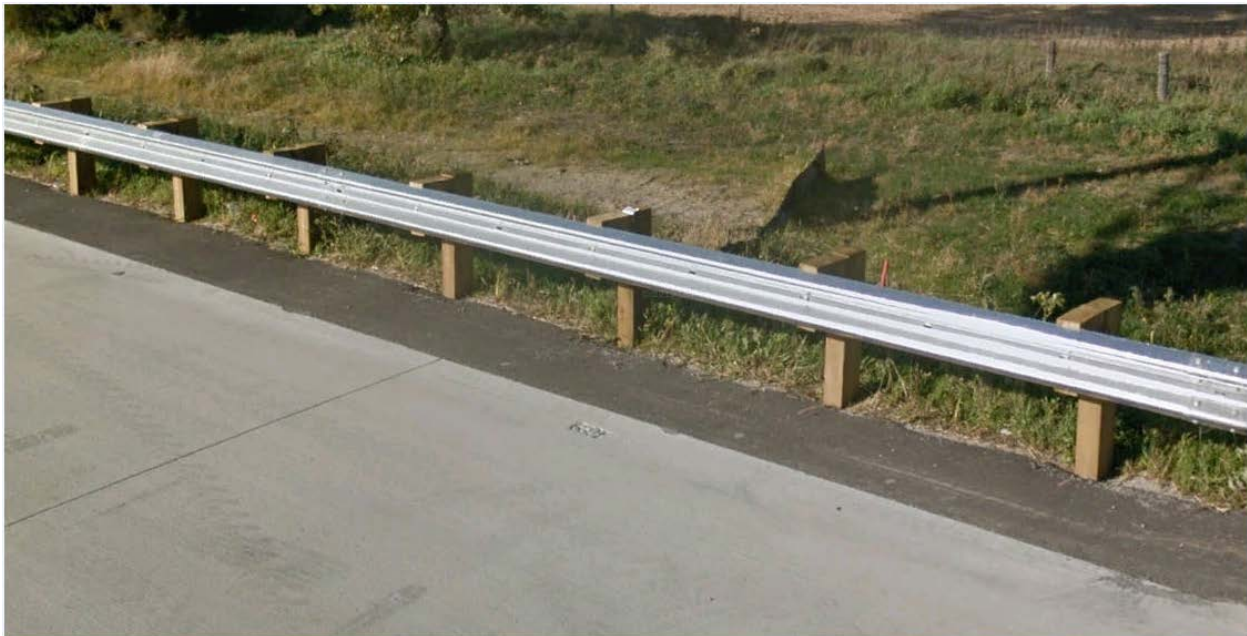
Figure 1: Steel beam guardrail.
