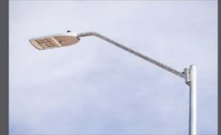
880 new tower and street lights
