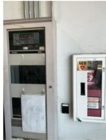
Alarm control panel
