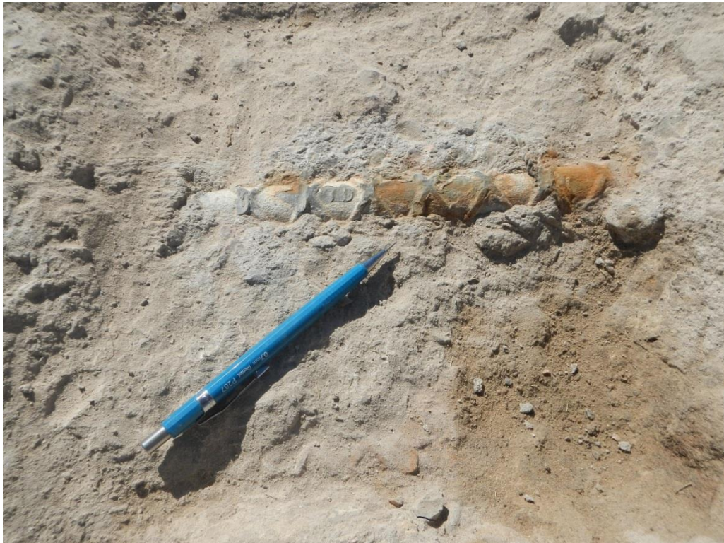
Figure E12. Close-up of corroded bar in westbound lanes.
