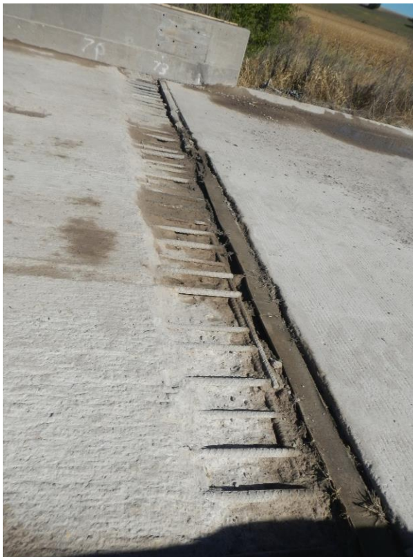
Figure E4. Deeper removal along end joint at westbound lanes
