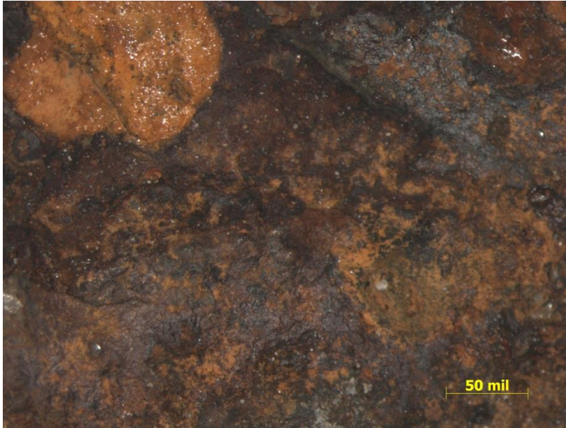
Figure 17. Micrograph of the top surface of Sample 10, showing red corrosion product from the steel.
