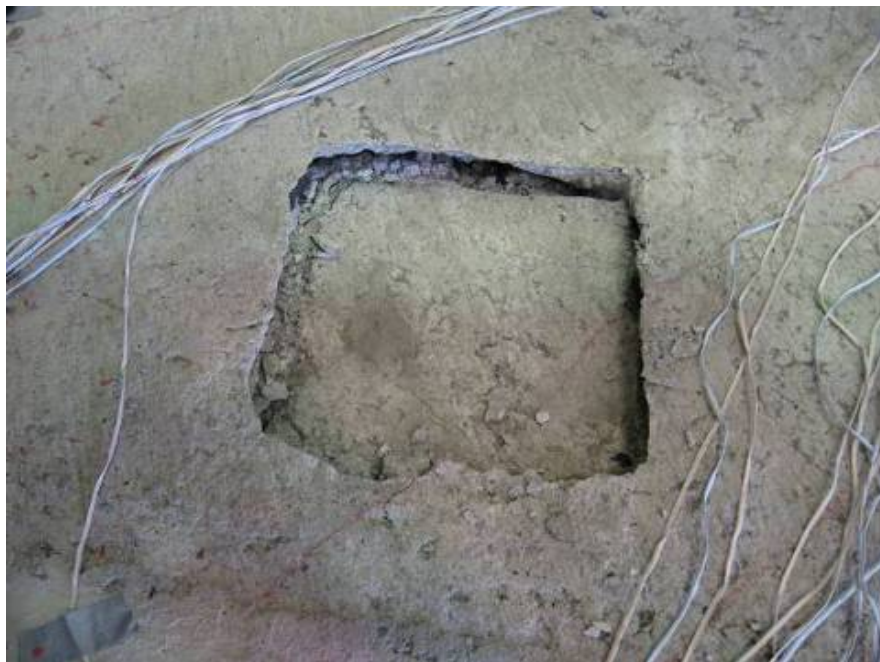
a) Top view of punching shear failure footprint
