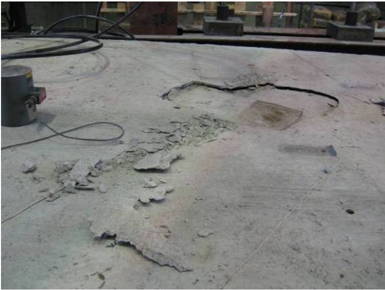
Figure 3.27. Punching shear and flexure failure due to tandem wheel footprint
