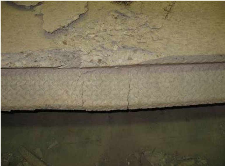
b) Flexure cracks
