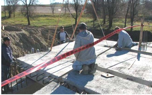
Figure 132. End panel being placed at the east end of the bridge, November 8
