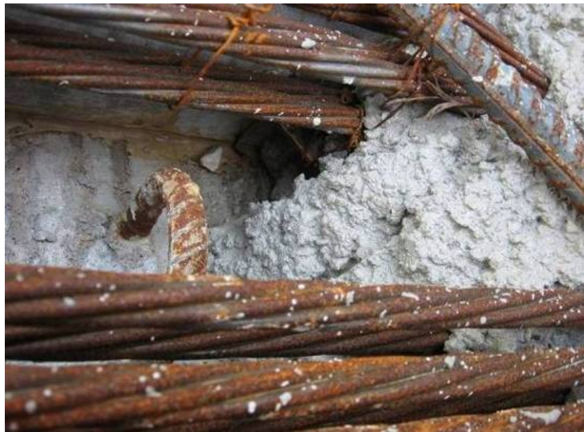
b) Concrete flowing between post-tensioning strands
