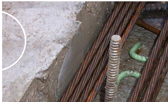
Figure 86. Concrete obstruction in Channel 1
