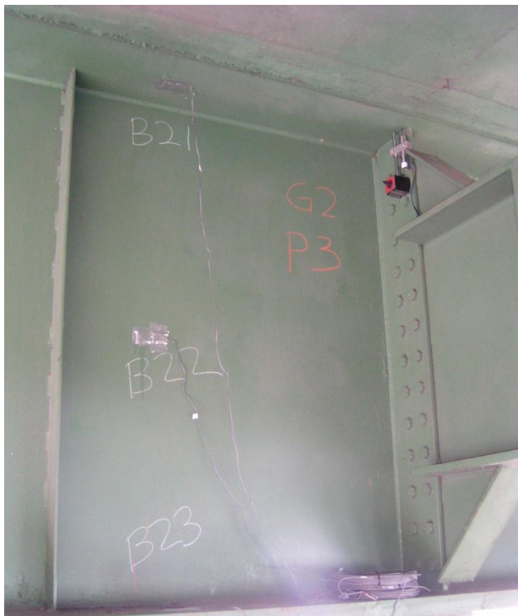
Figure 22. Strain gages B21, B22 and B23 on Girder 2 to assess flexural behavior near Pier 3.
