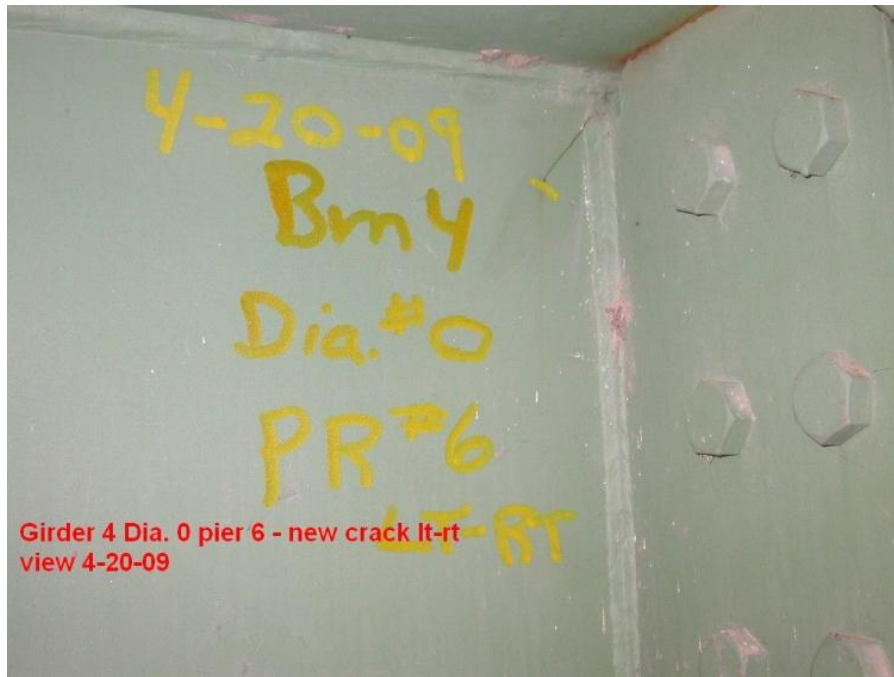
Figure 5. Fatigue crack on Girder 4 at Pier 6 of westbound I-80 Bridge over the Cedar River. The 2 ½ in. crack was found in April 2009.
