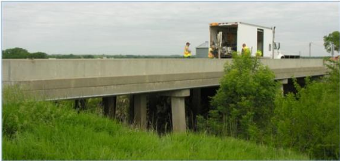
Figure 104. Side view of Deck O6 showing continuous slab construction on east face.
