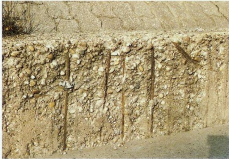
Figure 6. Crumbling and scaling of a concrete surface after freeze and thaw cycles (Nuernberger, 1995).
