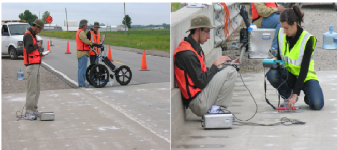
Figure 108. PSPA and GPR (left), PSPA and electrical resistivity (ER) data collection near south abutment in NB lanes.
