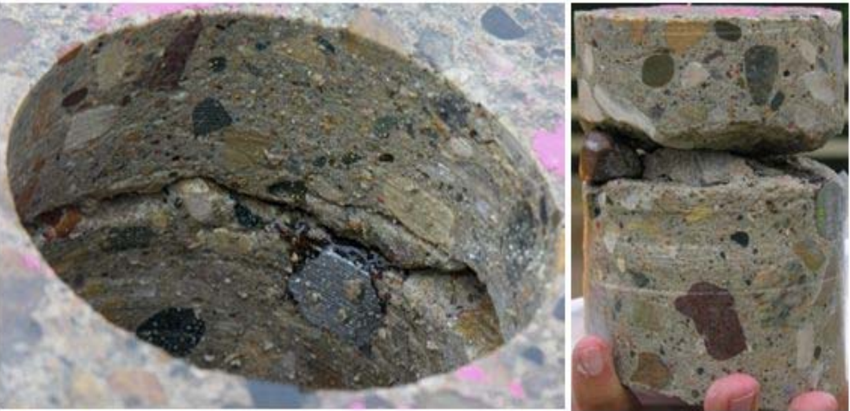
Figure 93. Hole and core sample (Core #3) with severe delamination and corrosion at top and sides of rebar.
