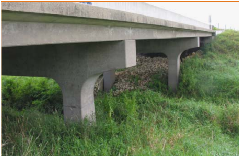
Figure 116. Side view of Deck R1 showing continuous slab construction on east face.
