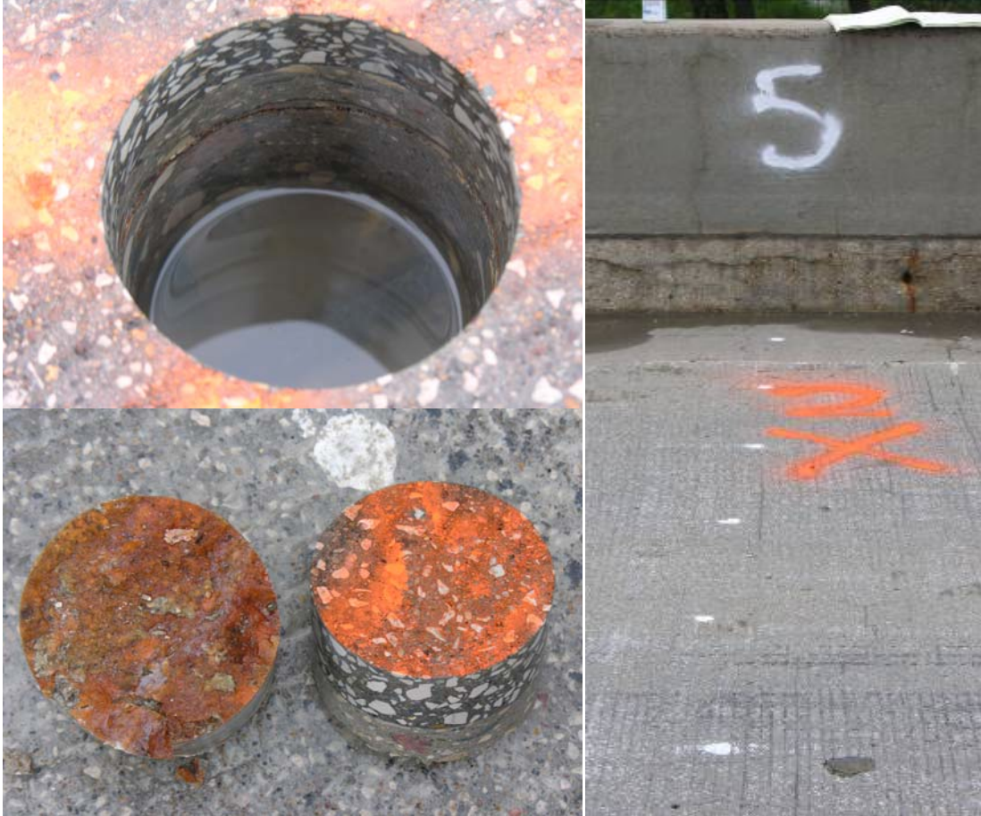
Figure 62. Photos of Core #2 location, showing extracted core, epoxy-filled delamination in core hole, and bonded overlay.
