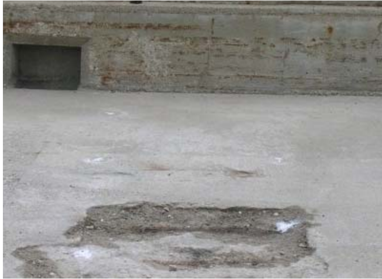
Figure 78. Surface spall exposes rebar, simplifying half-cell preparation (equipment not shown).
