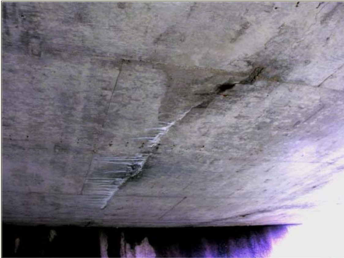
Figure 117. Bottom view of Deck R1 (continuous slab) with rust staining, efflorescence and crack running between pier and abutment.
