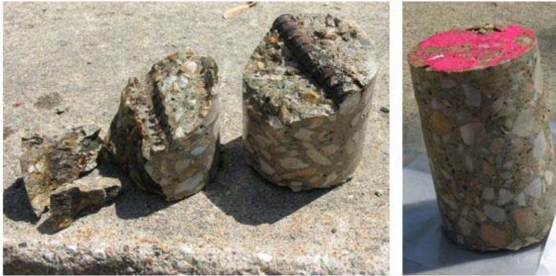
Figure 73. Cores #3 (left) and 4 (right), selected as “deteriorated” and “control” (sound) specimens for Deck O2.
