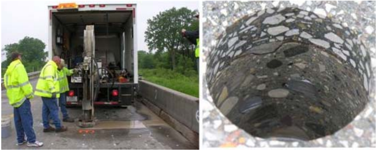
Figure 67. Core # 3 during extraction, where upper edge of delamination meets the debonded overlay just below the overlay, with both longitudinal and transverse rebar seen in the photo.
