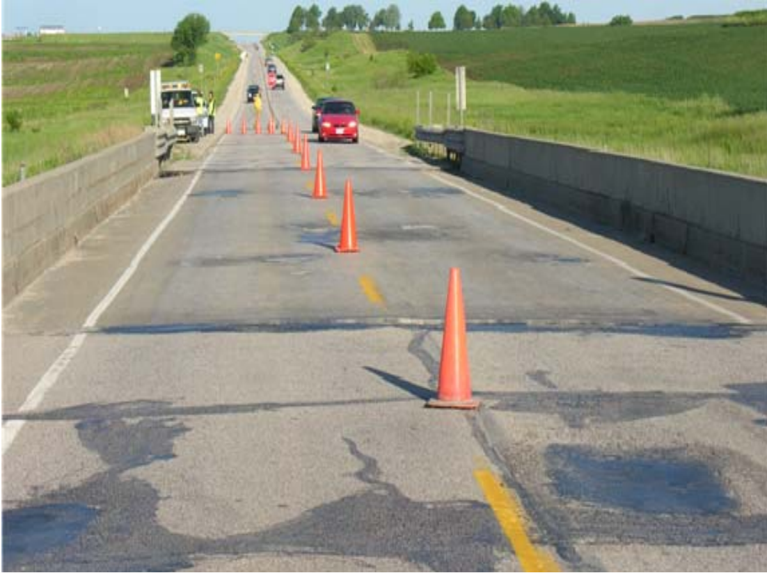
Figure 96. Perspective view of Deck O5, showing patches and spalls; also, repaired settlements in approach slab (foreground).
