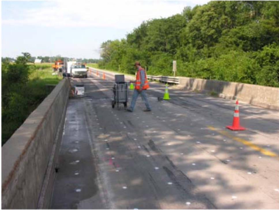
Figure 134. Perspective view of Deck R3, looking SW down northbound lane of Iowa #1.
