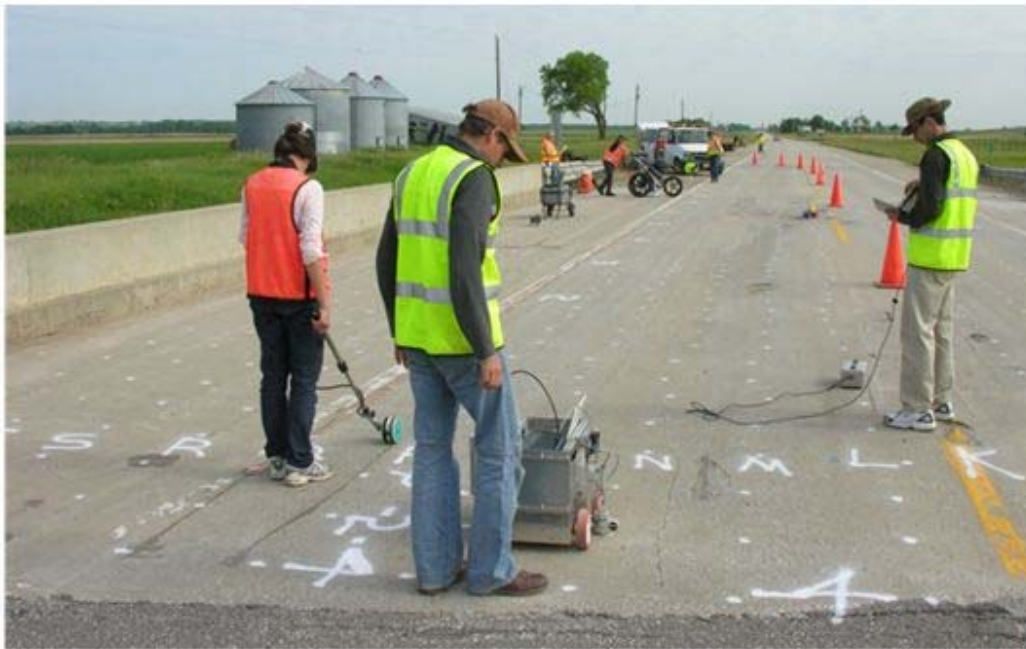
Figure 106. Multiple NDE methods collected in longitudinal direction on SB lanes, with GPR data collection across lanes.
