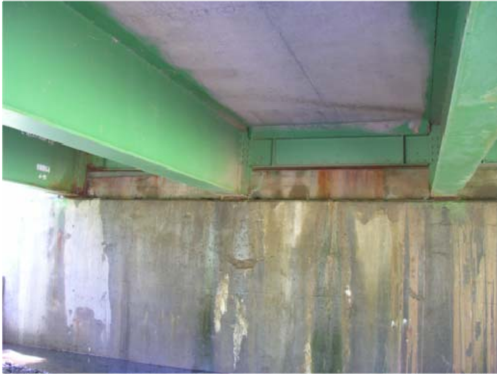
Figure 136. Bottom view of Deck R3 with rust staining, cracking and efflorescence at abutment.
