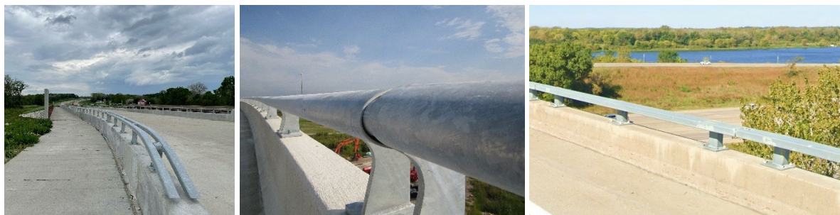
Figure 9.5.11.1-1. Examples of unpainted galvanized steel traffic railings
