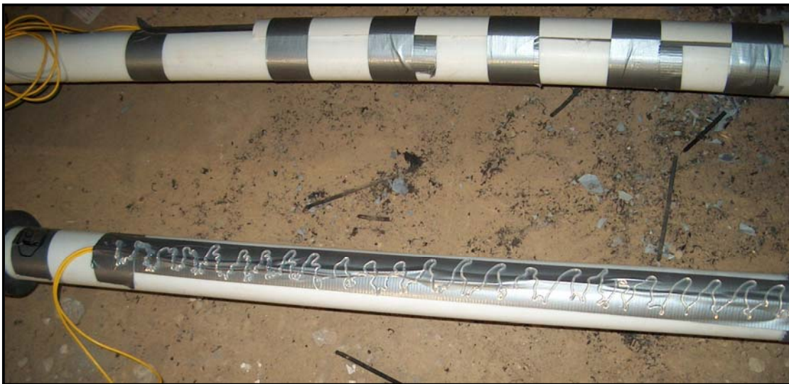
Figure 3. Improved sensor protection system used at 40 th Street Bridge
