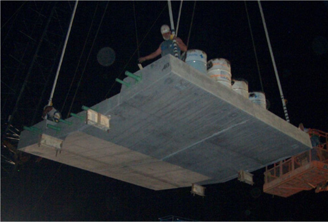
Figure 10. Sand-filled barrels used as ballast during erection of 40 th Street Bridge panels
