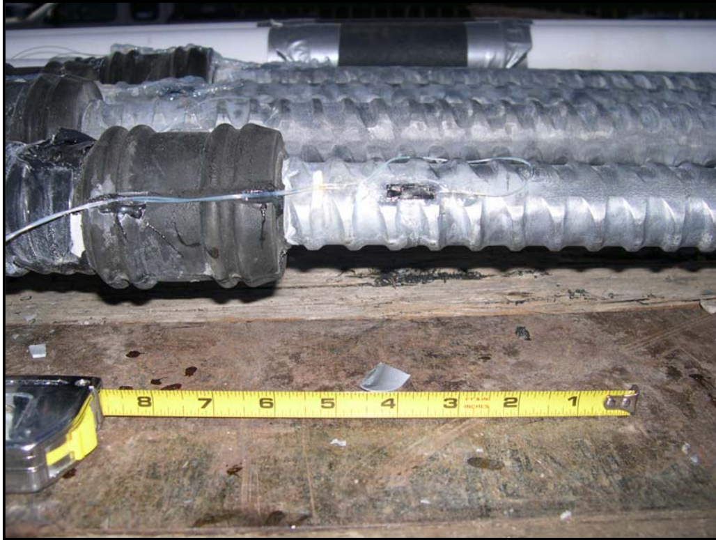
Figure 1. Fiber optic sensor attachment to hanger rod
