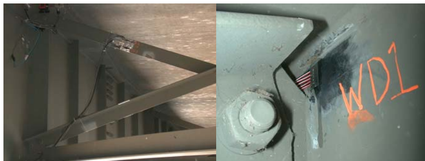
FIGURE 7. Photographs of Diaphragm and Web Gap Strain Gages
