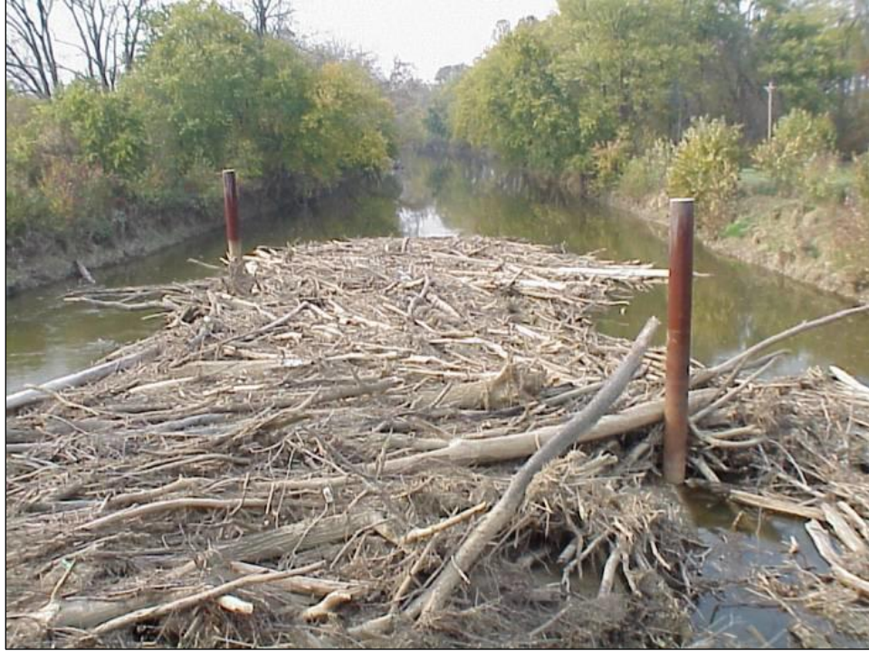
Figure 14. Debris accumulation at single column debris deflectors (Lyn et al. 2003)
