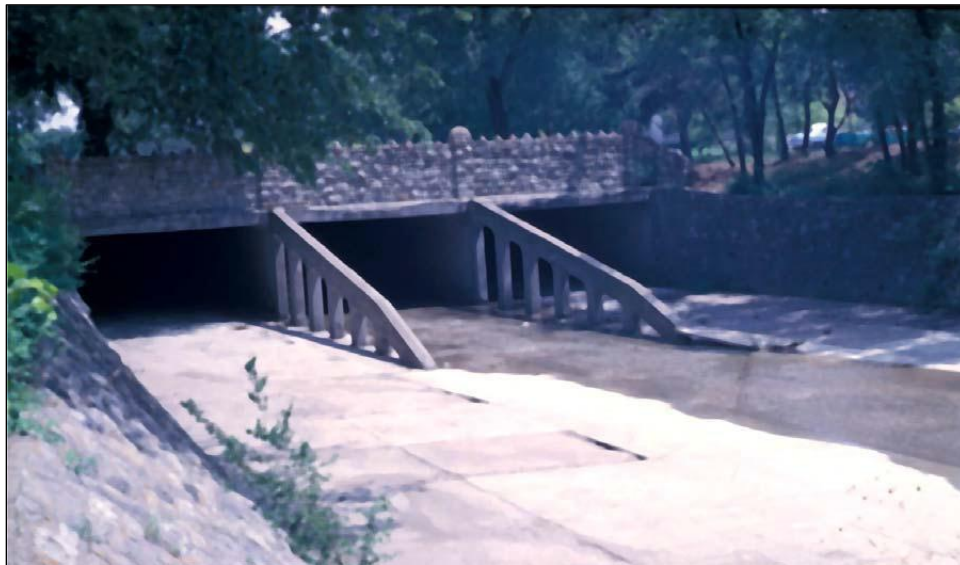
Figure 1. Debris fins upstream of bridge piers (Lagasse et al. 2010)
