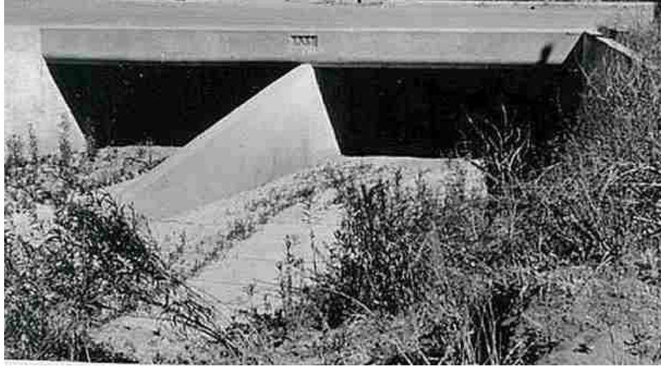
Figure 2. Debris fin upstream of bridge pier (Bradley et al. 2005)
