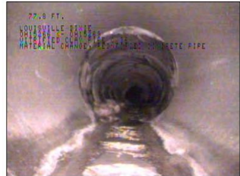
Photo: OH15269_OH15266124720_05112009_A.JPG, VCR No.: FLOOD WALL#2, 01:45:49 77.8FT, Material Change, Reinforced concrete pipe
