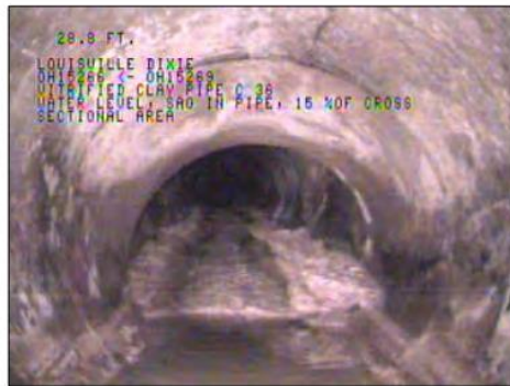
Photo: OH15269_OH15266124455_05112009_A.JPG, VCR No.: FLOOD WALL#2, 01:43:58 28.8FT, Water Level, Sag in pipe, 15 %of cross sectional area
