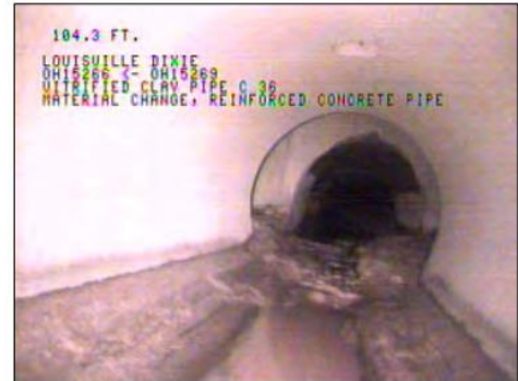
Photo: OH15269_OH15266124907_05112009_A.JPG, VCR No.: FLOOD WALL#2, 01:46:54 104.3FT, Material Change, Reinforced concrete pipe
