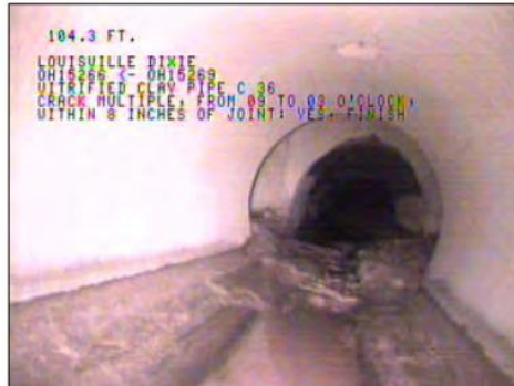
Photo: OH15269_OH15266124848_05112009_A.JPG, VCR No.: FLOOD WALL#2, 01:46:48 104.3FT, Crack Multiple, from 09 to 03 o'clock, within 8 inches of joint: YES, Finish
