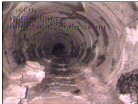
Photo: OH15269_OH15266124748_05112009_A.JPG, VCR No.: FLOOD WALL#2, 01:46:07 83.6FT, Material Change, Vitrified clay pipe
